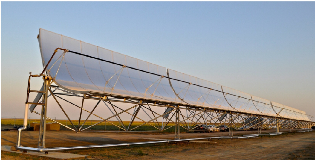
Fig. 3. The large parabolic trough solar thermal concentrator used to power the AHP–MED desalination process.
